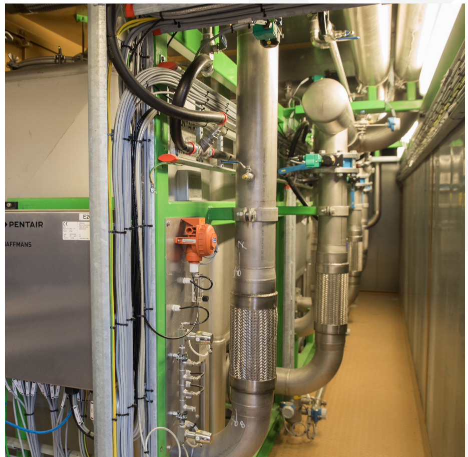
Activated carbon filtration
