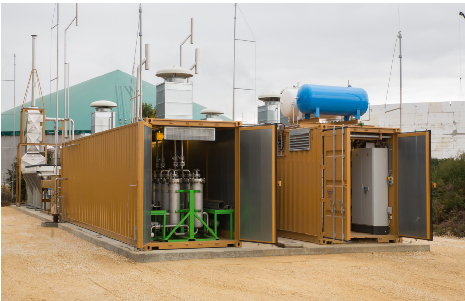
Pentair Haffmans Biogas Upgrading System
